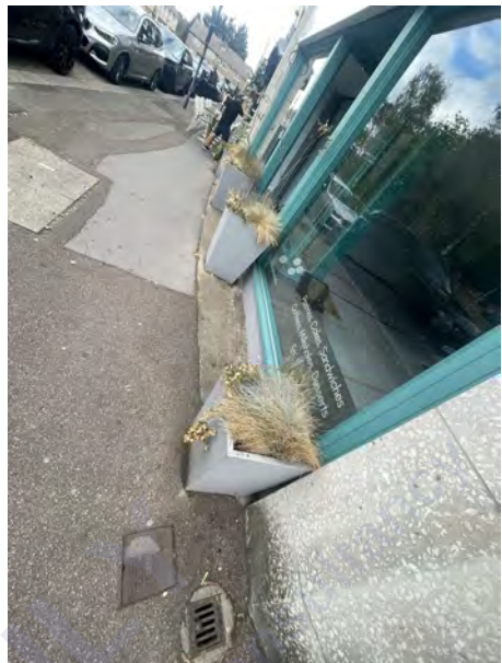
Plate A6 Two of the planters standing against the shop front glazing, with dead and dying planting.
