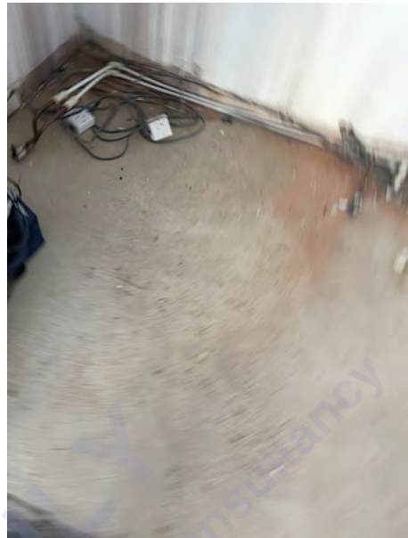
Plate H6 The base of the rear room wall, with staining to the lining and discolouration to the floor at the corner.
