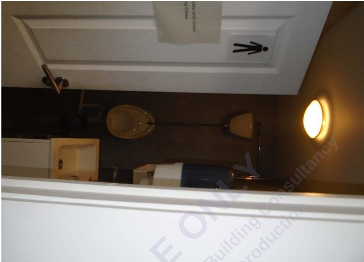
End of Schedule of Condition
